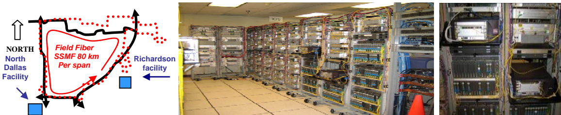
Fig. 1. Verizon 80 km loop, Xtera 3040 km all-Raman ULH system, Mintera 40Gbps transponders.
